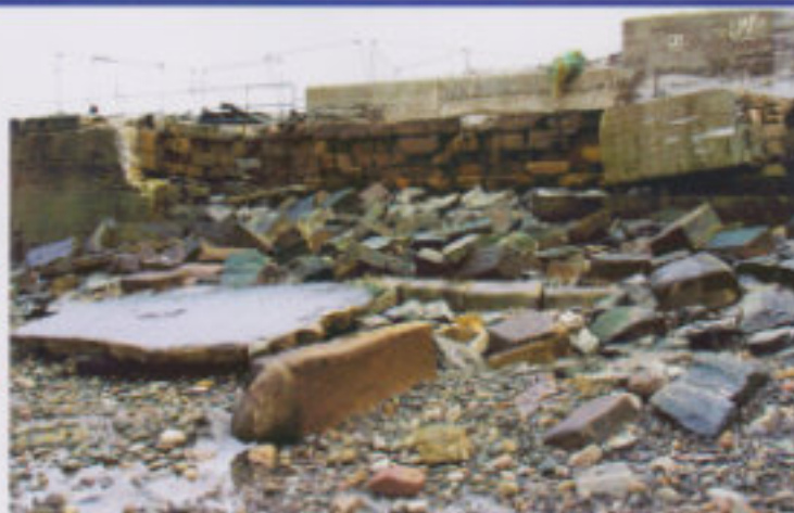
Following the huge damage caused by the December storm, high water and big waves in February caused further falls of masonry and brought fresh fears.
